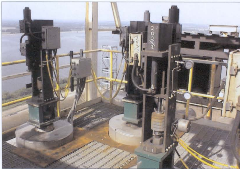
Left: Three of the four superheater bypass valves replaced at a 750MW Babcox and Wilcox Universal Pressure Boiler supercritical plant in Kansas, USA. The effect of the valve replacement work saw one of the largest one-time improvements ever seen in a power plant.
