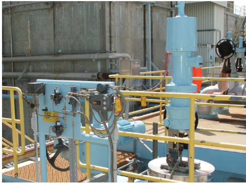
Feedwater regulation valve with panel mounted instrumentation
