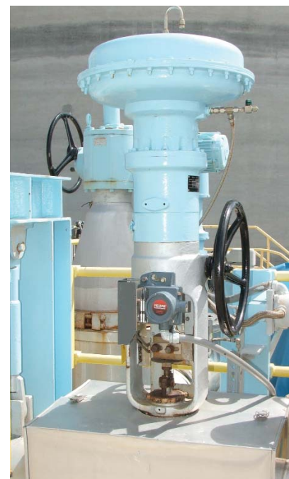
Feedwater bypass valve with remote mounted feedback sensor
