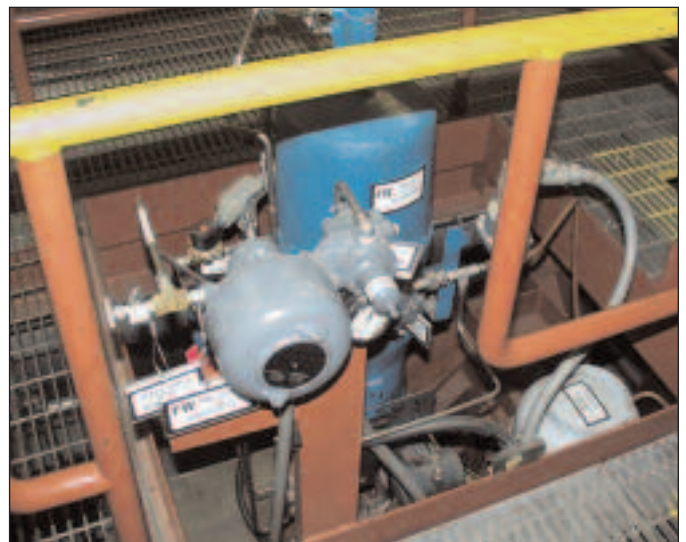
Figure 3. Original installation, I/P transducer and actuator
