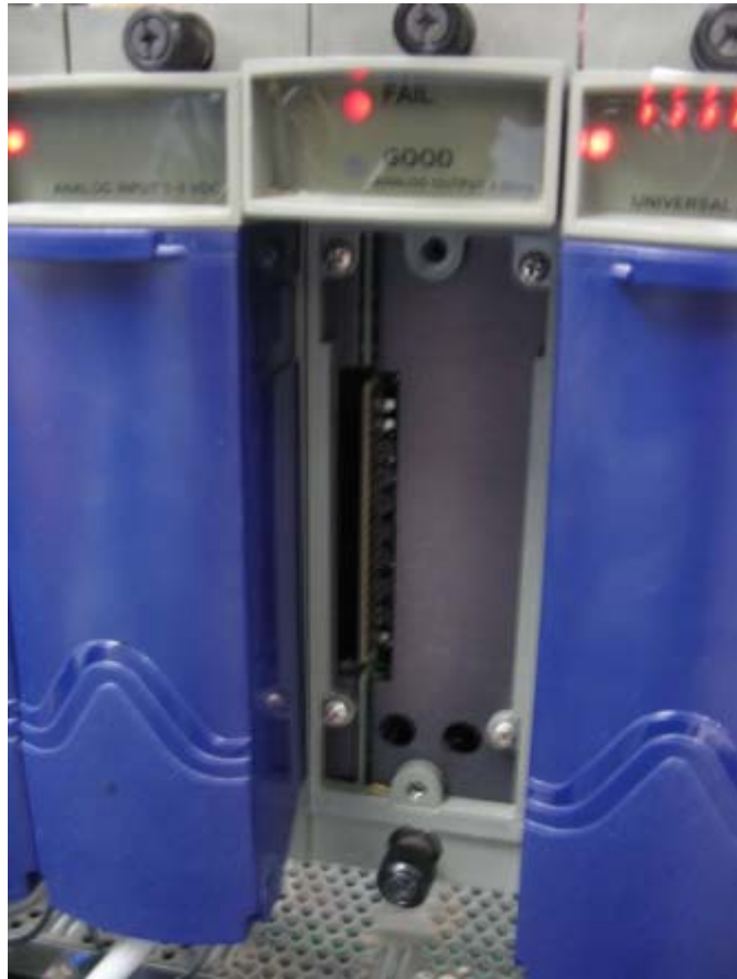
Figure 5-9. New I/O Module in Place Prior to Attaching Terminal Board and Terminal Housing Assembly
