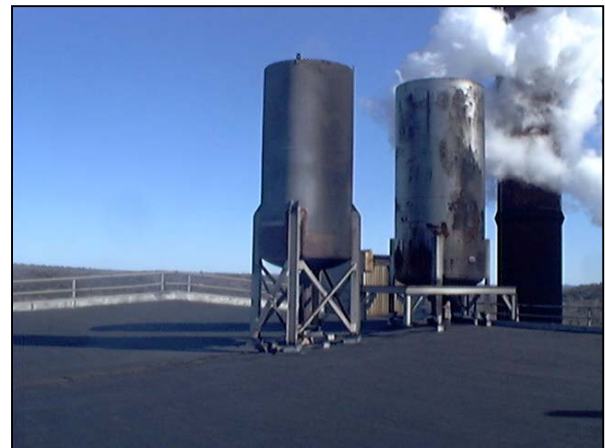
Figure 2: Existing Silencer Arrangement
