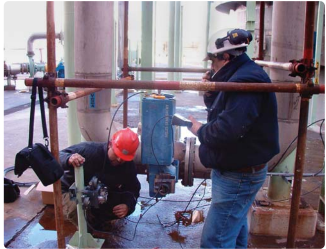
Two instrument technicians, one from INECO (red hat) and one from CMPC-Pacifico (white hat), used a handheld device to calibrate a new FIELDVUE® instrument installed on a valve in the filtrate lines at the base of the pulp mill's consistency tower.
