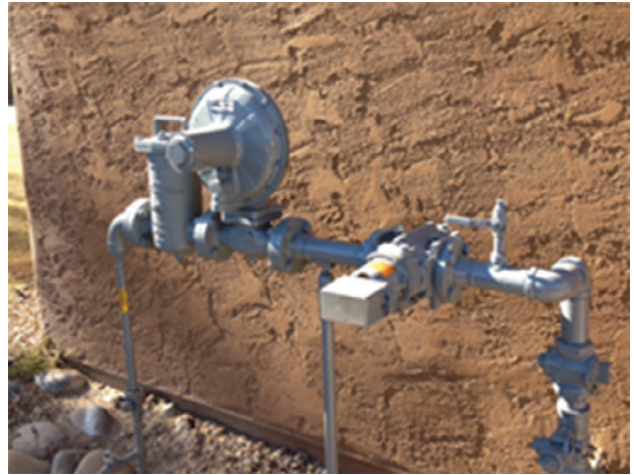
Figure 2. Commercial Meter Set
