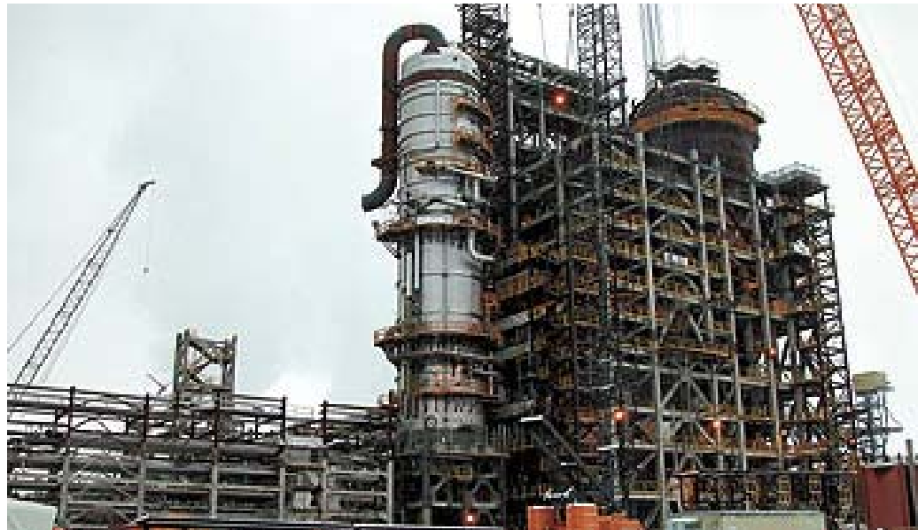
Coker 8-3, above, is part of Syncrude Canada's Upgrader Expansion Project. Emerson's AMS Device Manager "will cut instrument commissioning time at least in half, which will amount to significant savings for Syncrude", said project consultant Gil Hurtubise.
