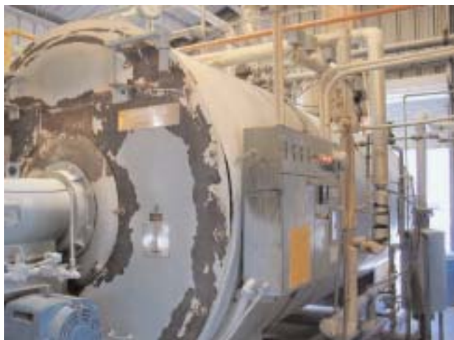
The McIntyre Ga. facility's process steam boilers use as much as 20,000 cu ft per hour natural gas.
