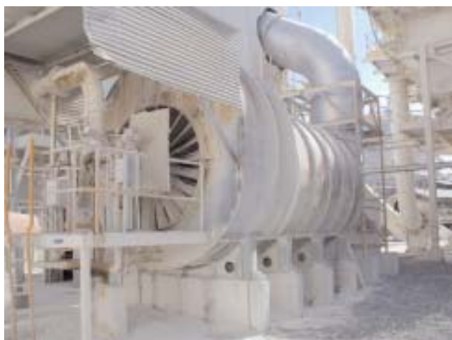
Burners used in drying operations require between 6,000 to 90,000 cu ft per hour natural gas.
